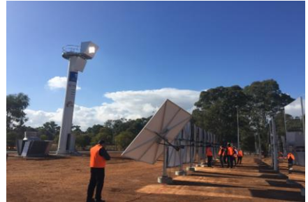
A solar field showing heliostats and a central tower
